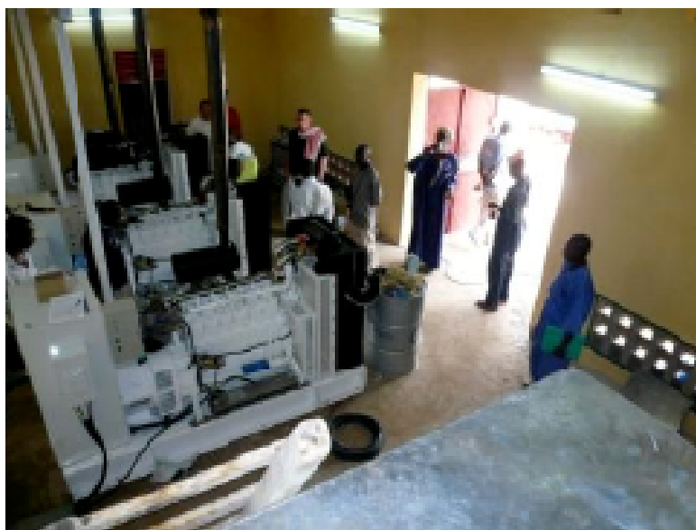
The new diesel electricity generator is launched in Garola
