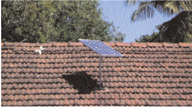
A small photovoltaic installation on a roof-top in India SELCO
